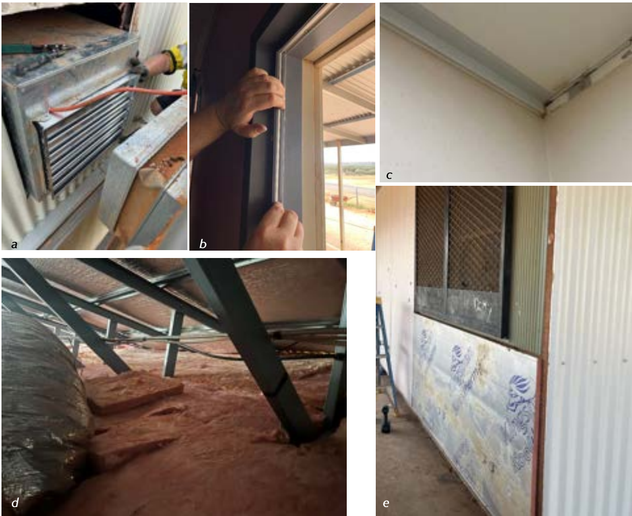
Figure 8. Examples of airtightness upgrades and thermal bridging mitigation measures: (a) damper installed in evaporative cooling system; (b) door seal; (c) new cornice detail, applied to linings with caulking; (d) semi-rigid glasswool covering roof truss bottom chords; (e) rigid foam board added to external walls.
